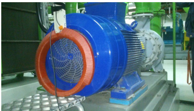
Figure 3. The axial flux measuring coil mounted during testing of a large machine
